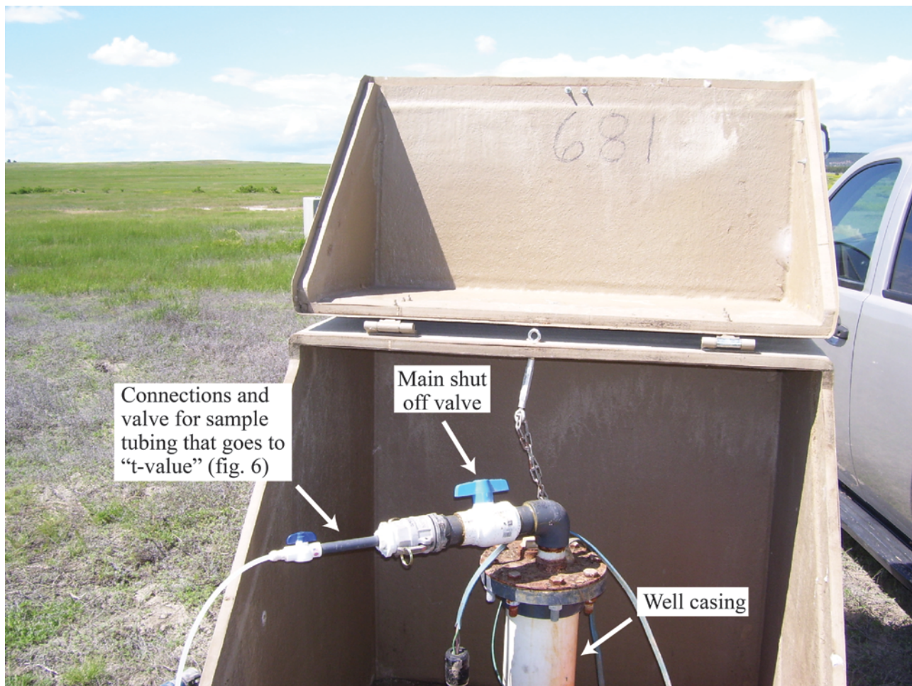
Figure 5. Typical wellhead control valves.
